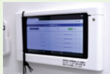
Visualizing energy consumption on monitors (energy management system (EMS))
